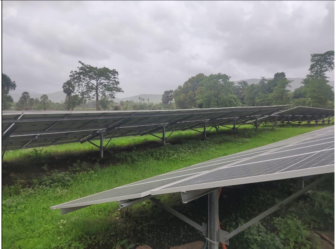
150 KW Solar Power Station
